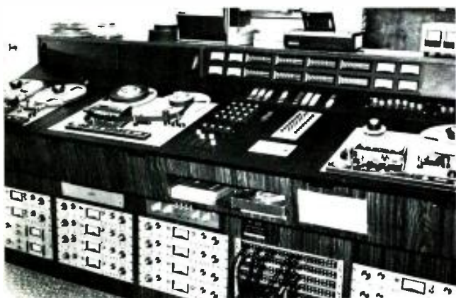
Superscope's custom mastering equipment includes Scully transports, Dolby noise-reduction units, Langevin Graphic and Audio Design equalization modules, Universal Audio limiters, and Allison Research Kepex modules.
